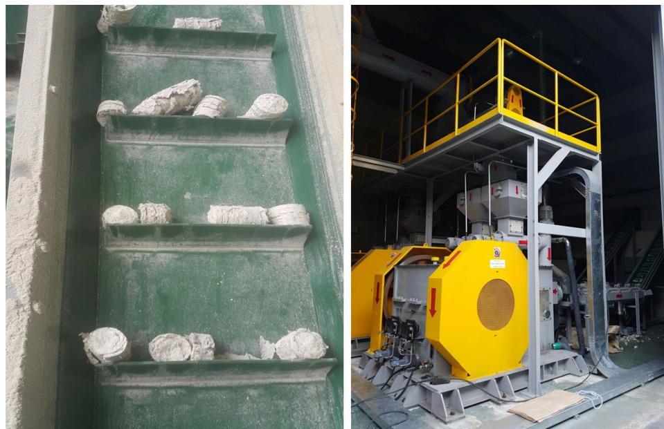
Fig. 4 Photographs of a polyurethane SRF product (left) and facility (right)
